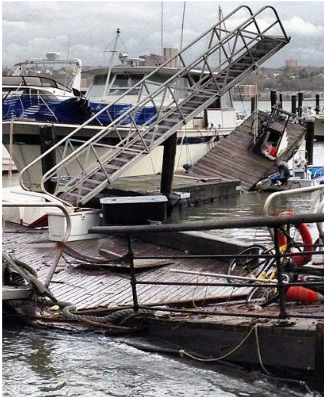
Dock & Gangway Damage
